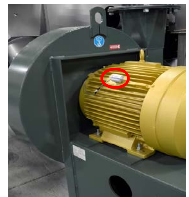
Fig. 1: Prophecy Sensor mounted on a blower
